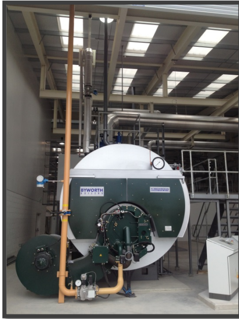
Complete Boilerhouse Installations
