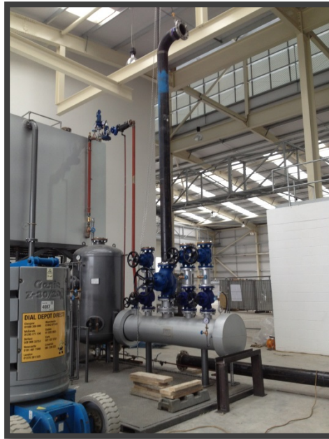
High/Low Pressure Hotwater Systems
